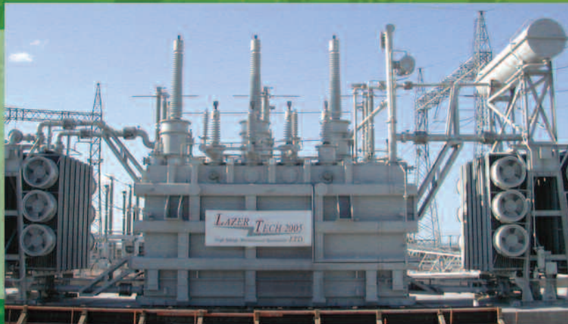
A 180MVA 275/66kV transformer recently relocated/overhauled/and commissioned for a major client in Adelaide, South Australia.
